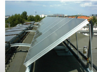
Installation on top of the building of Phönix Sonnenwärme AG
