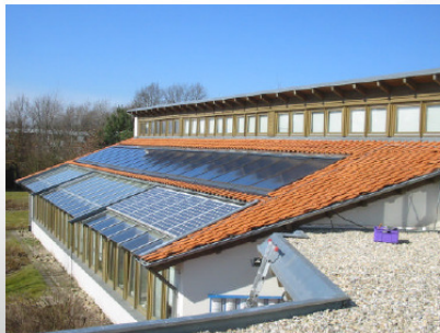
Installation, CUT Osnaabrück
