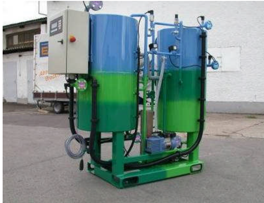
15 kW absorption chiller
