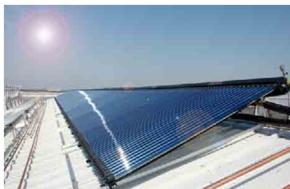
Figure 4: Evacuated tube collectors at Venice Marina (picture source: Climatewell)
